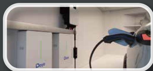
Smart EV Charger
