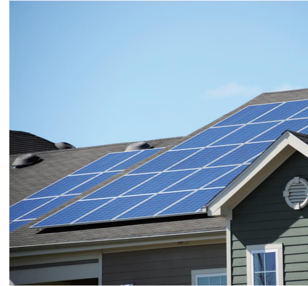
Residential Project in Indonesia 6kW
