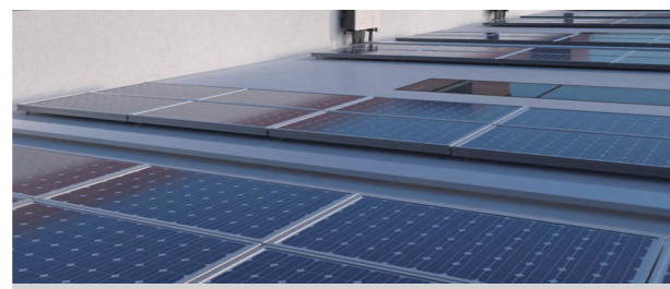
Residential Project in Poland 3kW
