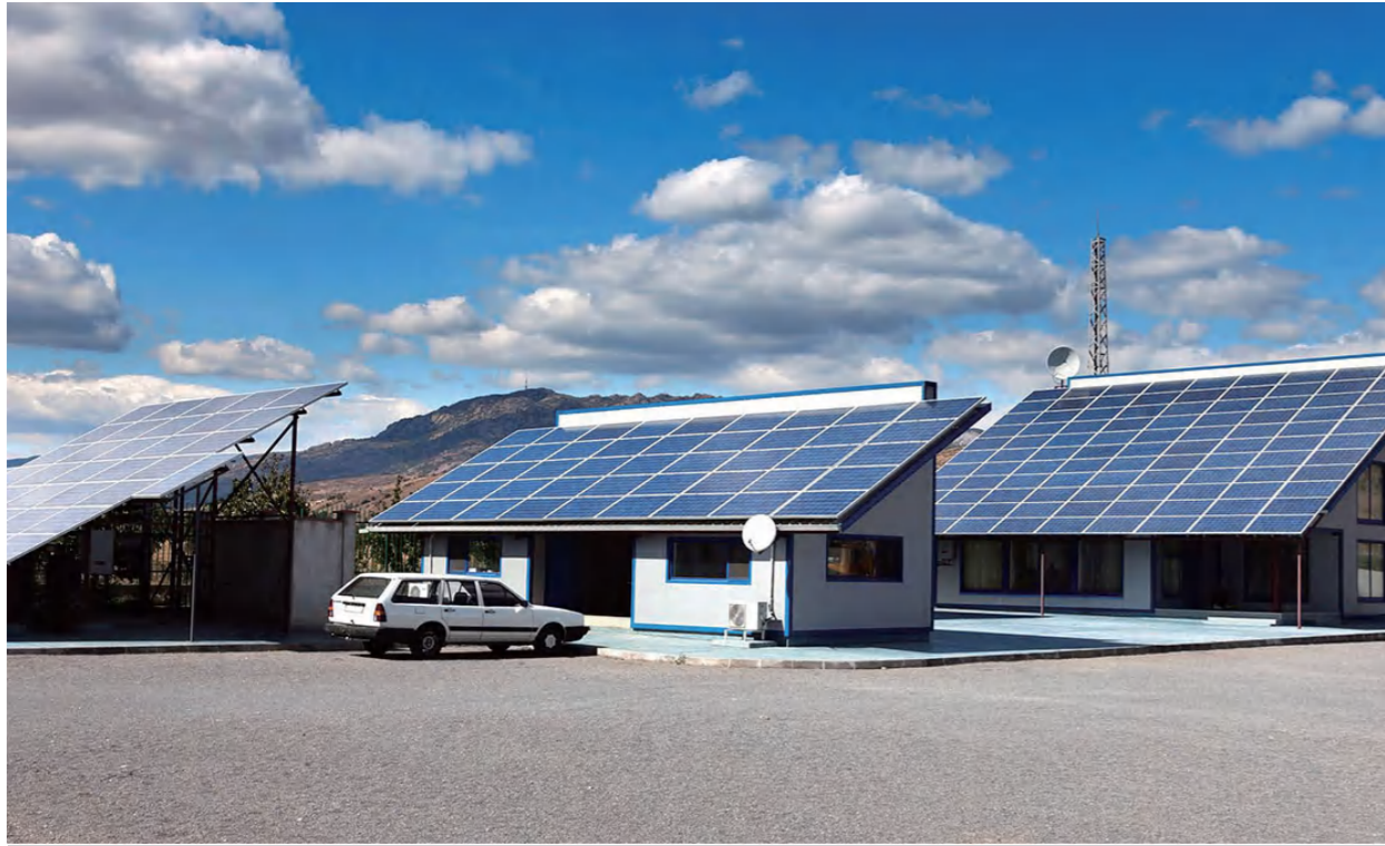
Residential Project in Indonesia 6kW
